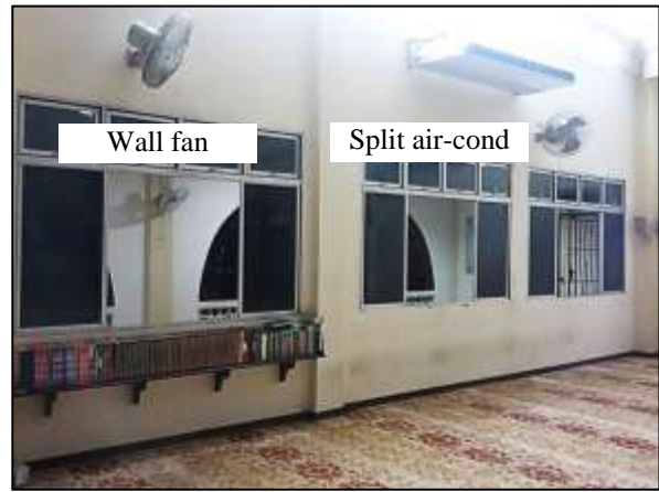
d) View of wall-mounted A/C unit and fans
